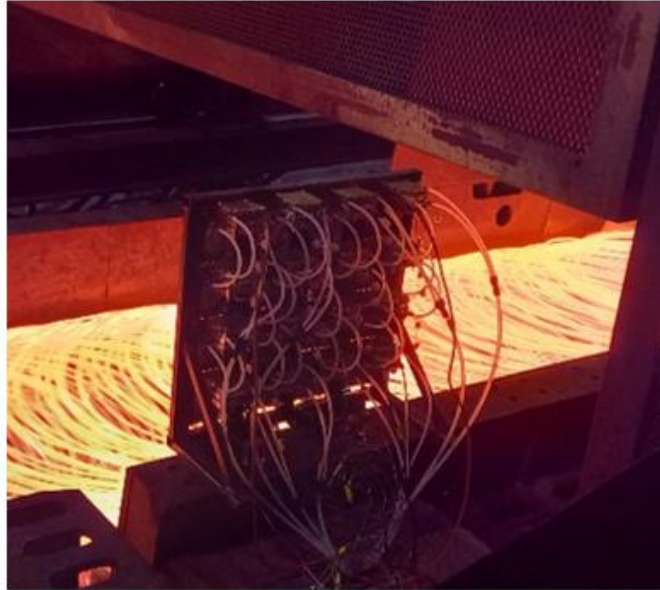
Installed WHP-Prototype at the hot wire rod mill of ESF site
