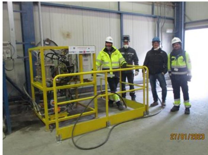
Prototype A installed at Ferriere Nord Osoppo plant
