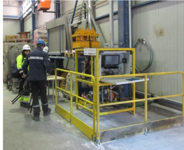
Prototype A – Installation and long-term trials of TEG tubes at Ferriere Nord steelworks
